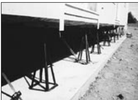
Once the home is leveled on jack stands, tie downs (diagonal steel ribbons) are anchored to foundation.
