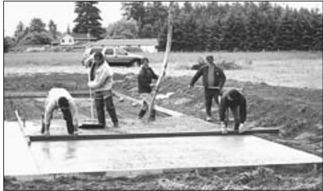
A worker (center) moves the end of the hose suspended from the boom of a concrete pump truck (not visible) to fill the form for a 6-inch deep foundation slab reinforced with 1/2-inch "rebar." The resulting "floating slab" will be given ten days to cure prior to the delivery of the home
